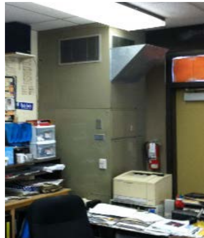
Inadequate HVAC Systems
